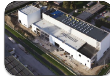
Neutral Beam Heating
